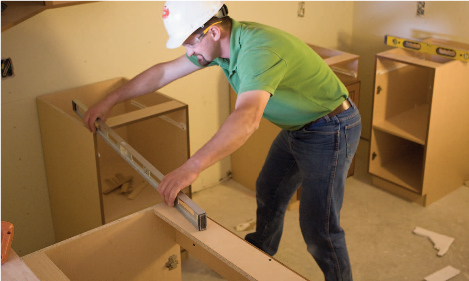
Installation personnel level cabinetry both horizontally and vertically to ensure a perfect installation of cabinets and custom fit wall fillers and scribes.
